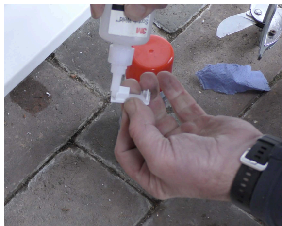
Attached the cill end caps using adhesive to seal and fix in place.
